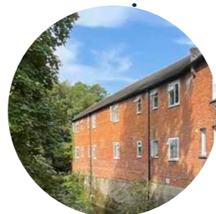
Long walls broken up by rainwater pipes
