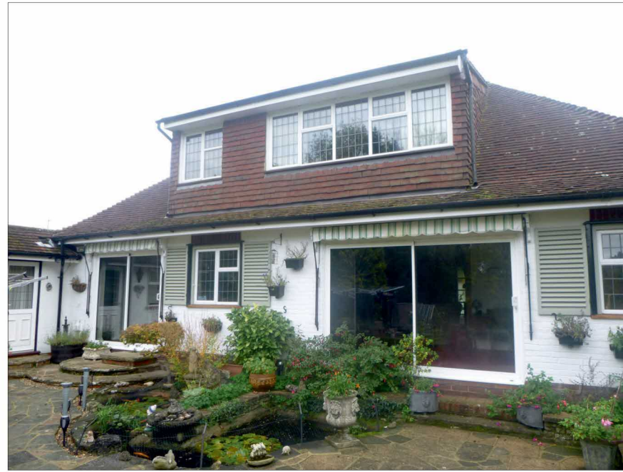
Photograph 2: Showing the rear of No.16 and area of tile hanging on the rear dormer.
