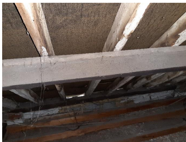
Plate 4.18: Gaps at Eaves, Light Entering
