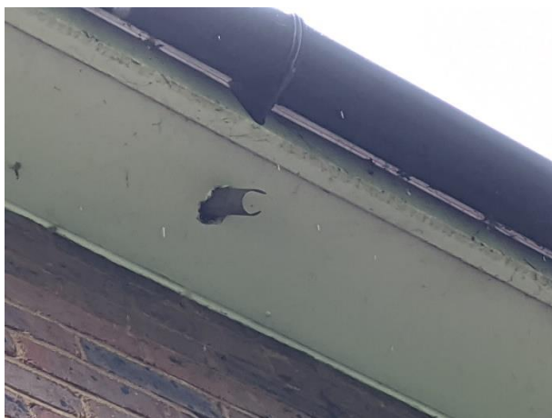
Plate 4.3: Gap Around Piping, Soffit Box, B1
