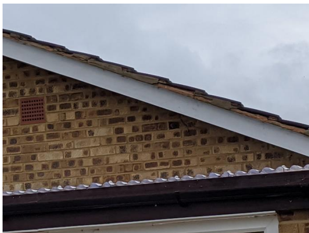
Plate 4.24: Missing Mortar, B7
