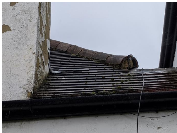
Plate 4.20: Lifted Lead Flashing & Missing Mortar, B6
