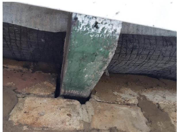
Plate 4.8: Gaps at Eaves, B2
