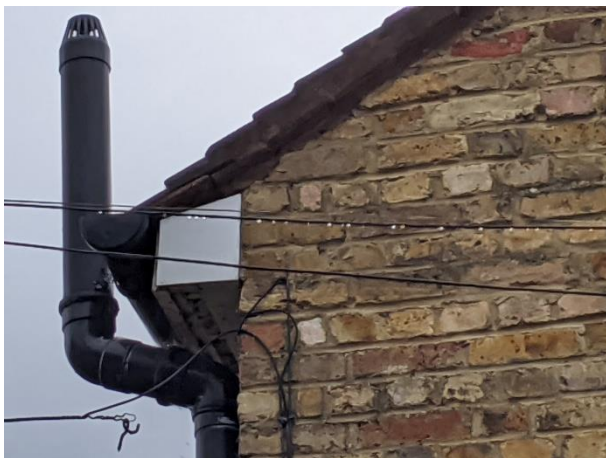
Plate 4.13: Gaps Around Soffit, B4
