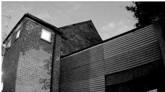
Photo 6: Screenshot of camera focused on the apex of Building 2 on the second Dusk emergence survey 30/06/2022
