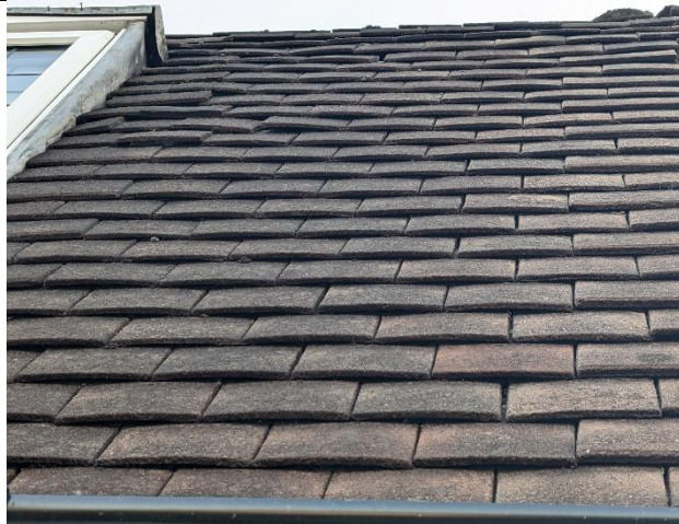
Photograph 3: Gaps beneath hanging tiles
