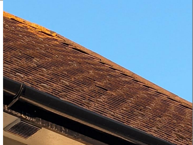
Photograph 4: Gaps beneath roof tiles
