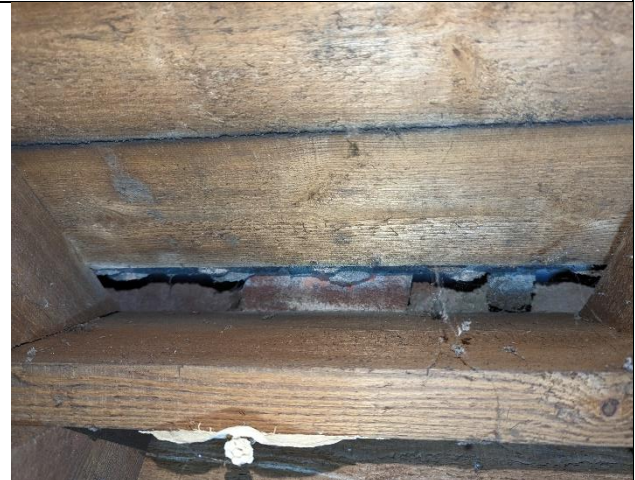
Photograph 6: Visible ridge cavity with cobwebbing
