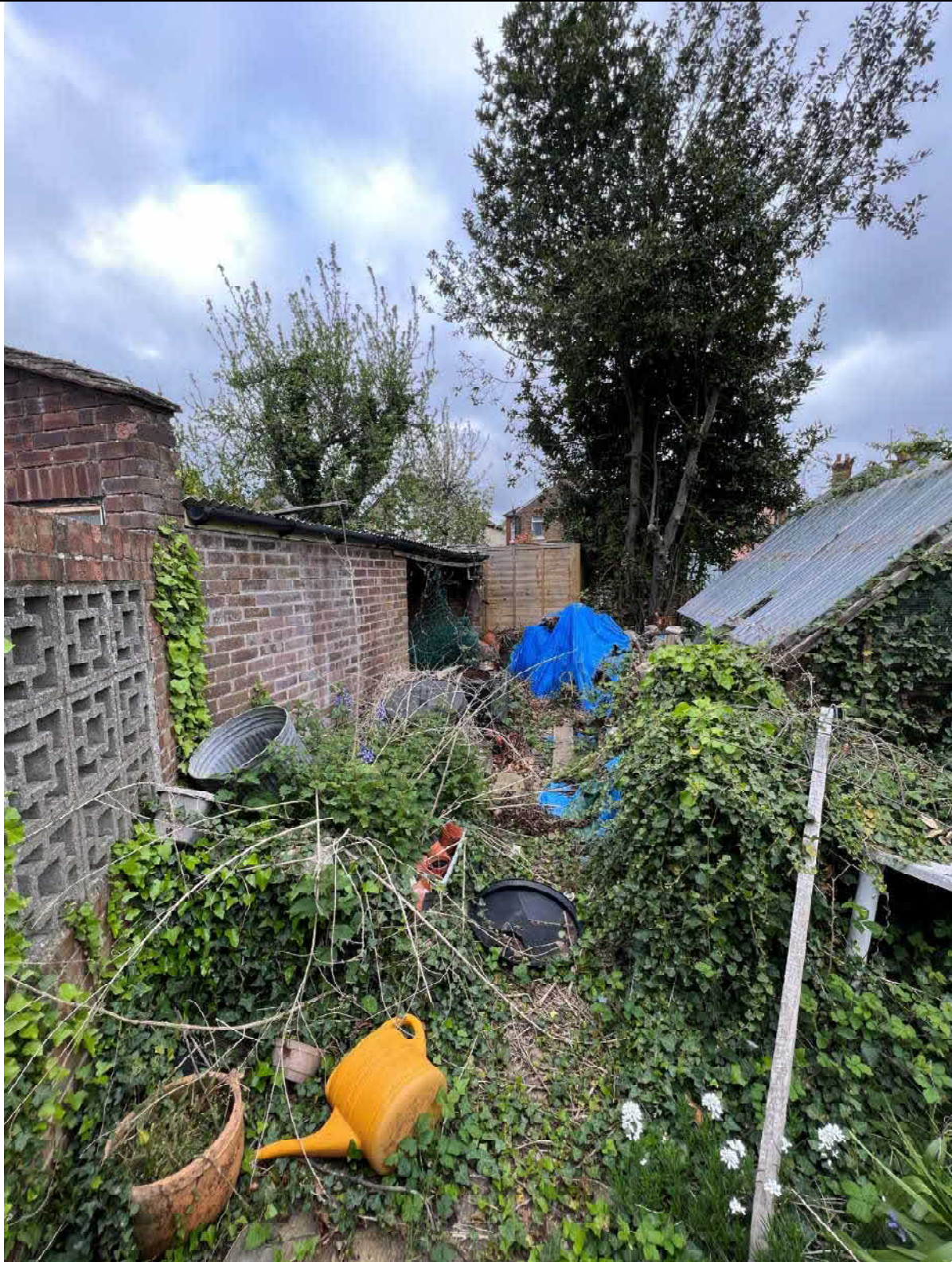
Photo 3: View of possible asbestos roofing.
