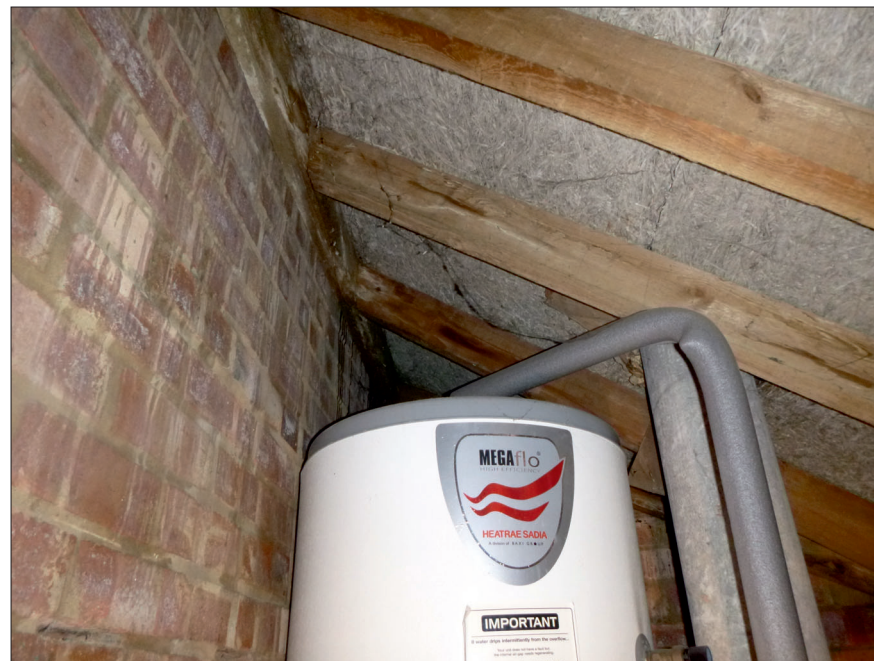
Photograph 4: Showing one of the service units' housing a boiler.
